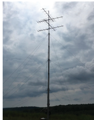
Figure 3b. A guyed, stand-alone tower array with two sets of quad-directional antennae.
