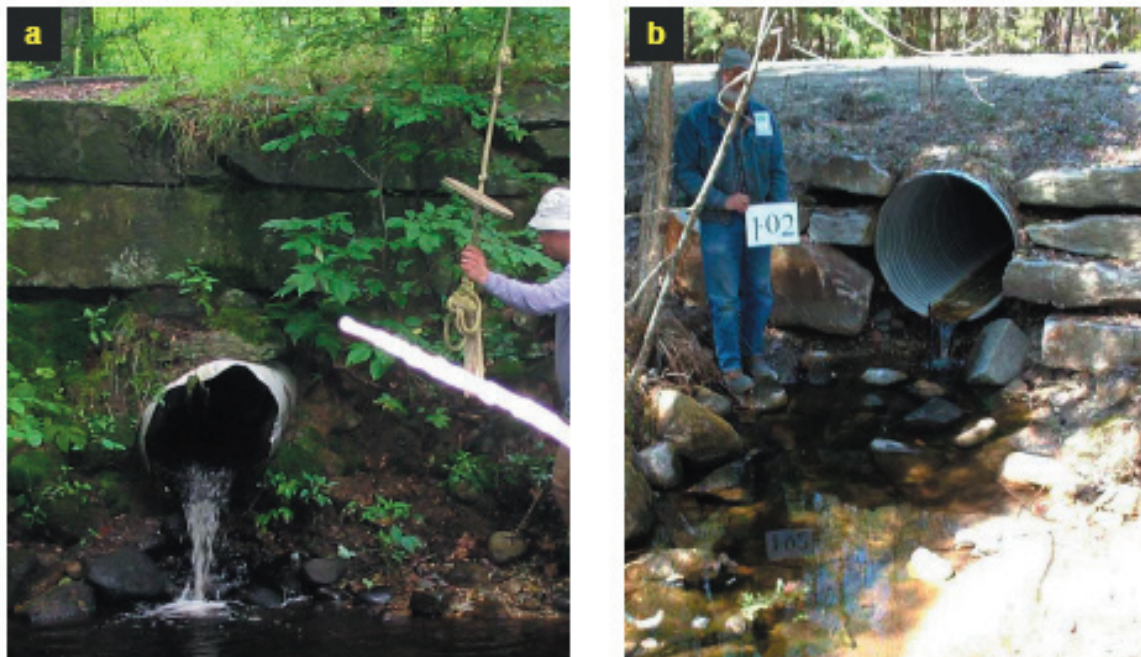
Images of "hanging" (a.k.a. "perched") culverts. Photo source: Maine DEP.
