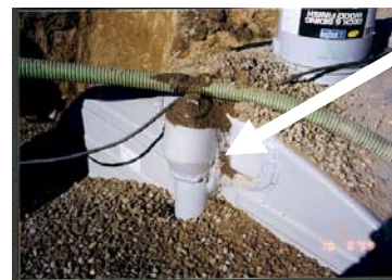
Upright tube in center is where the interstitial sensor is located.
