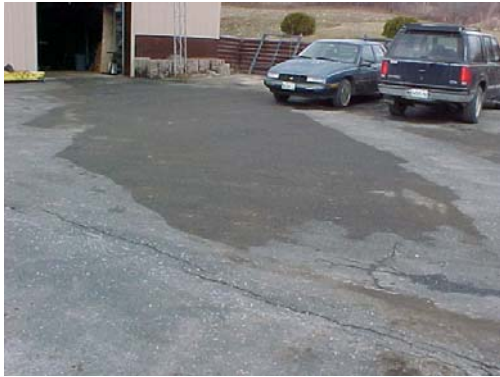
Cleaning up an overfill during delivery can be expensive
