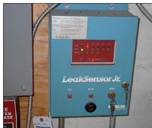
A leak sensor in alarm.
