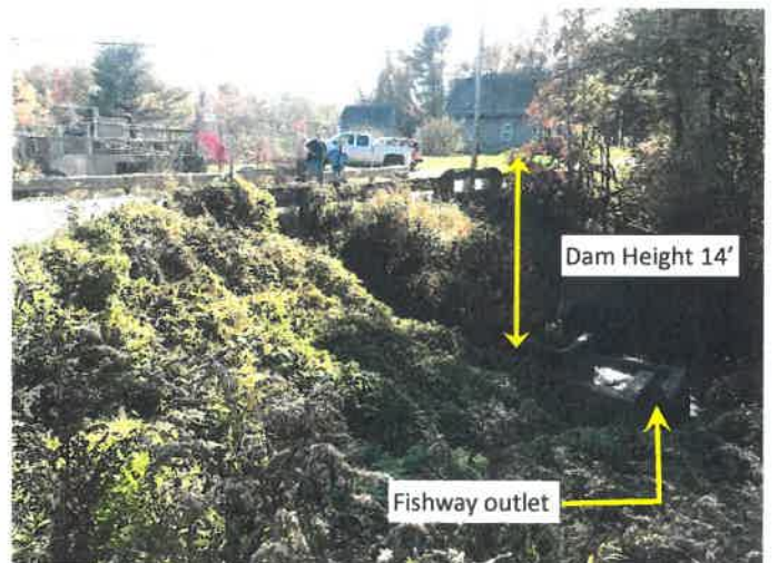
10. Downstream road embankment which merges with the road embankment. Fishway outlet lower right. Toe of dam assumed at channel outlet to bridge.
