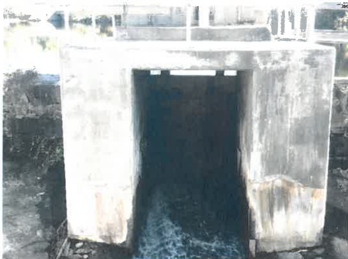
9. Concrete piers & slab housing sluice gate & electric hoist. Rust streaks are likely at construction joints.
