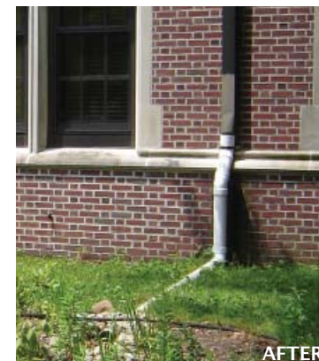
The image on the far left shows the approximate drainage area for a roof with more than one downspout. The two images in the center and near right depict both before and after the disconnection of the downspout from underground pipes.
