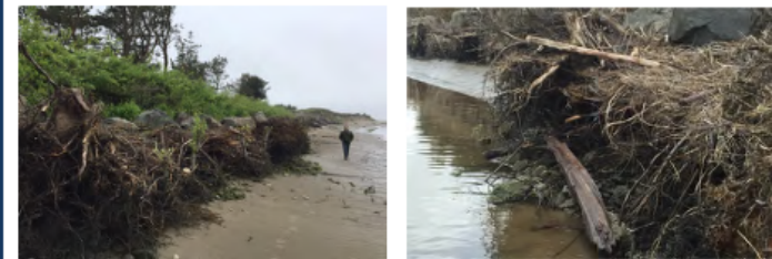
Figure 1. Root wads inserted into unstable banks can help protect bare soil from erosion, from a project in coastal Oregon. In areas not suitable for living shorelines, root wads can be an effective alternative providing stabilization and habitat.
