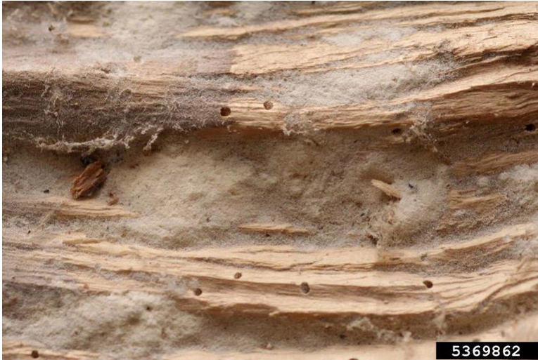
Wood damage from powder post beetles.
