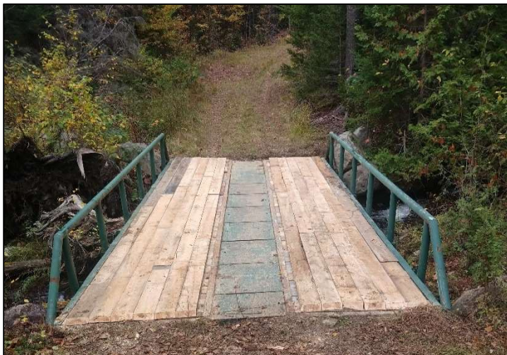
New bridge installed over Trout Brook at the Little Moose Unit, BPL Western Region
