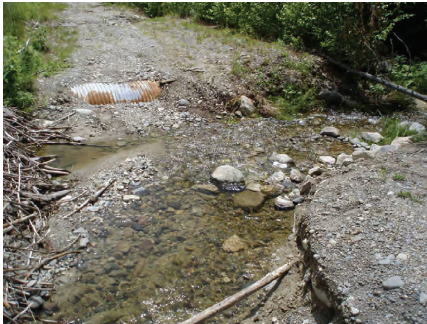
Flooded section of the 22-00-0 Rd.
