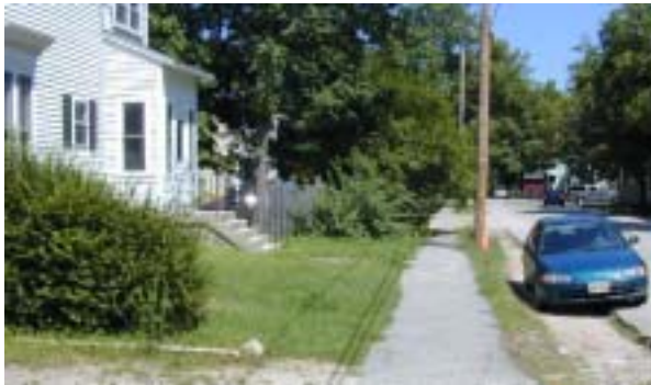
The esplanade has deteriorated to a point where curbing may be required.
