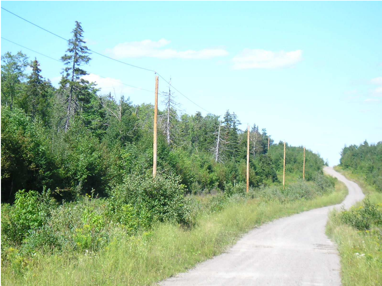
Utility Service Line
