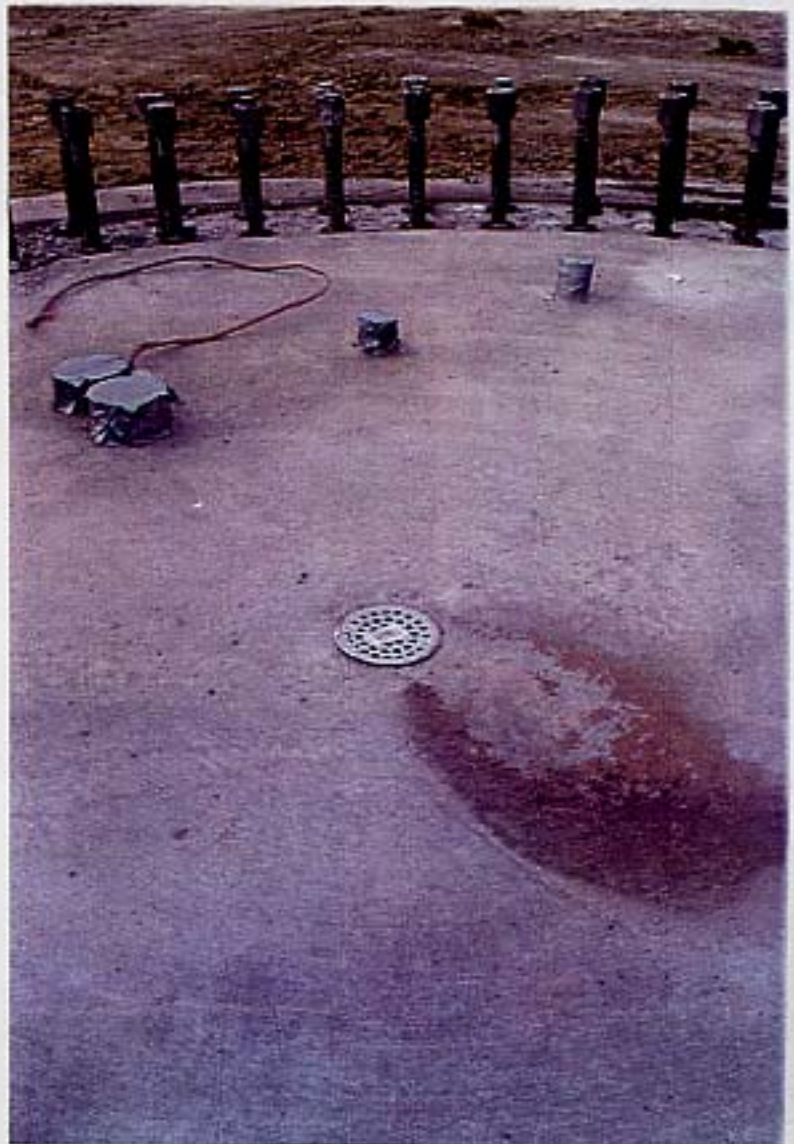
FLOOR ATOP FOUNDATION GROUNDING WIRE ELECTRICAL CONDUITS, COMMUNICATION CONDUITS, CENTRAL DRAIN GRATE
