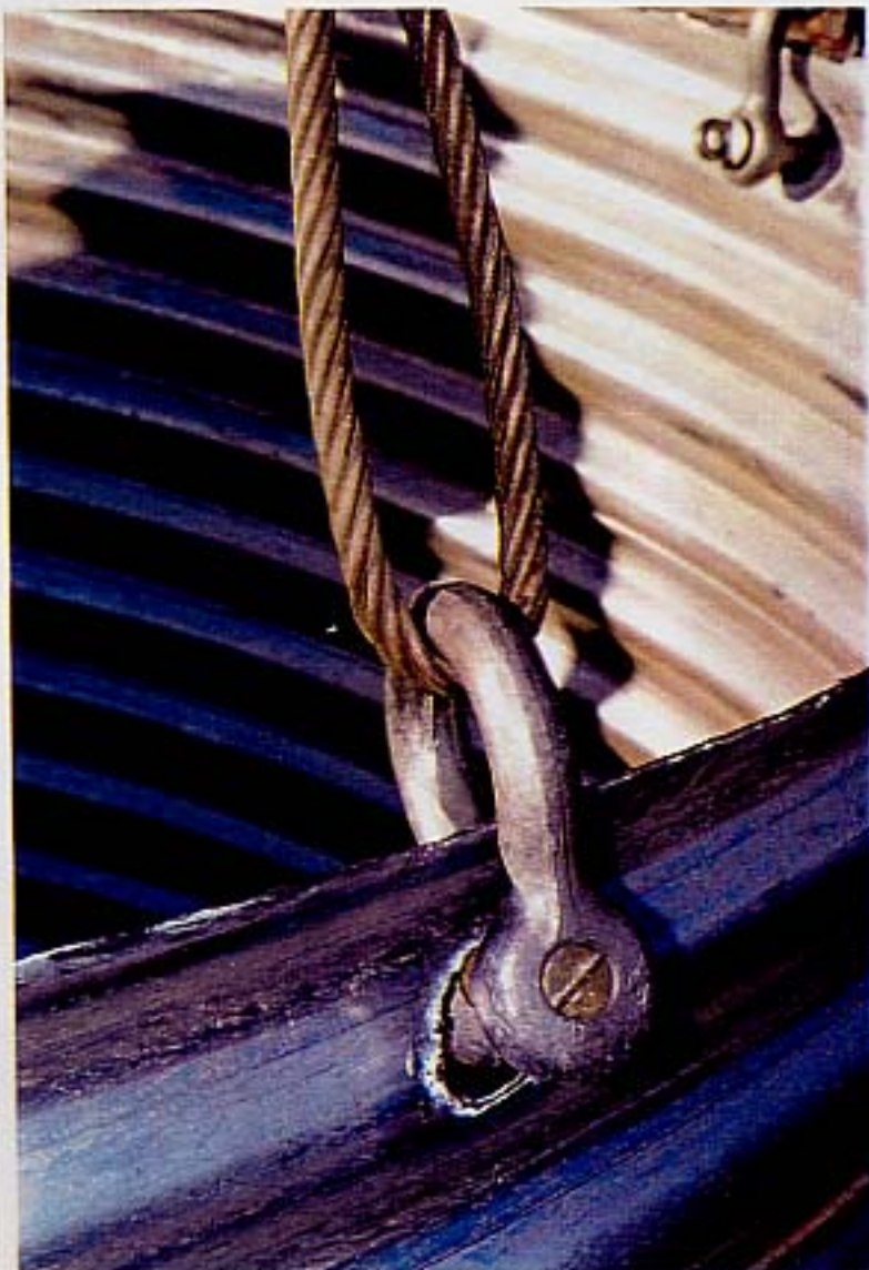
CRANE CABLE CONNECTION CMP
