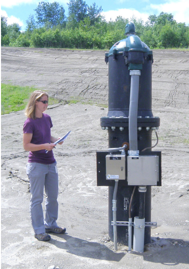
Municipal public water system inspector, Denise Douin, inspects Greater Augusta Utility District's well on a sanitary survey.
