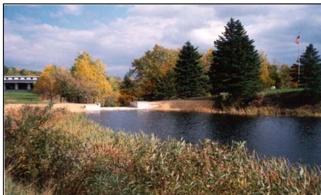
Construction of a stable, concrete dam outlet and repairs to a deteriorating causeway culvert served to decrease bank erosion, restore historic water levels, and improve fish habitat in Daigle Pond.
